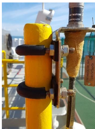
Figure 1 – Example of cable fixing
